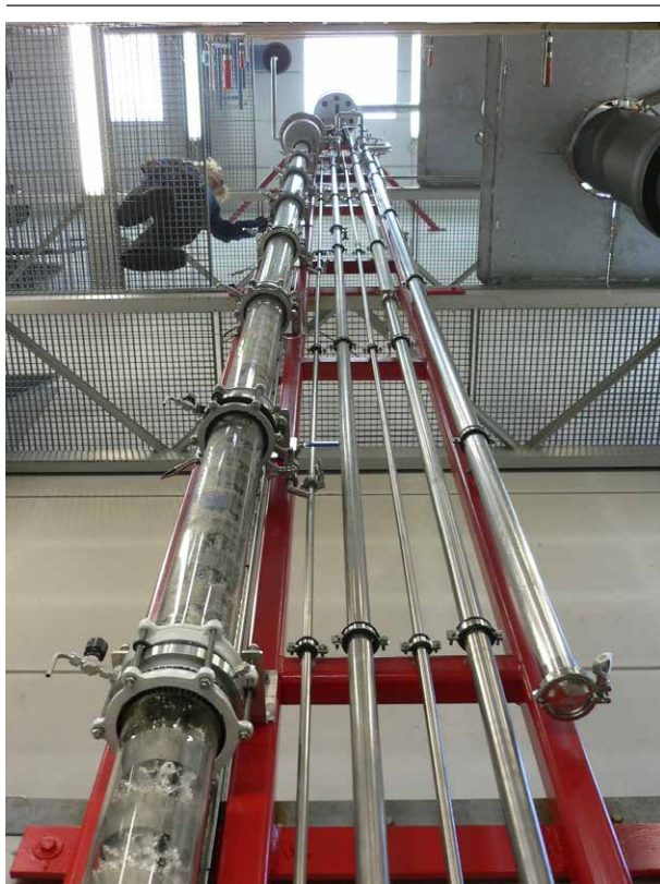
Figure 1. A view of the DTU absorption column
